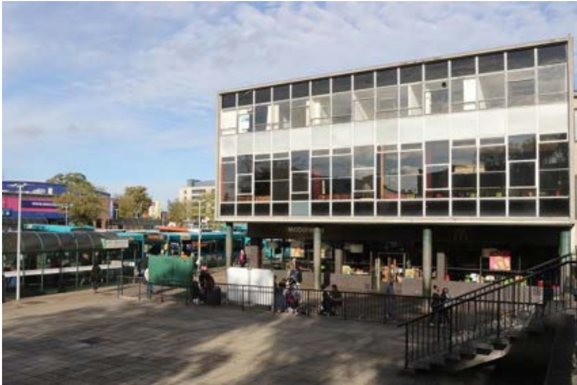
Figure 9: Stevenage Town Centre's North Block in 2015. The modernist architecture has been poorly maintained and the largely-unused stock rooms above the ground-floor retail units have resulted in the upper-storeys deteriorating further (Eastnews, 2015).
