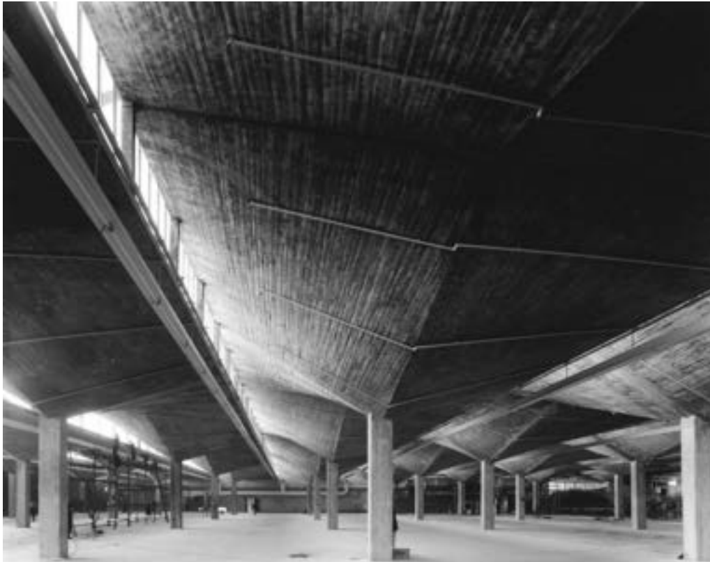
Figure 5: Grade-II listed warehouse in Stevenage designed by Felix Candela, his only UK work (Snoek, 1963).
