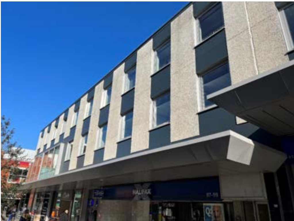
Figure 31: The west (above) and east (below) faces of Queensway. The west face is privately owned whereas the east is owned by SBC. The differing level of maintenance has resulted from the fractured ownership of the Centre following the dissolution of SDC in 1980. By maintaining as opposed to redesigning the façade, stakeholders further demonstrate their willingness to promote original New Town design. Furthermore, the west face demonstrates the updated canopy design incorporated in 1990. Historic England have described this as “highly intrusive” compared with the original (Cole & Harwood, 2020, p. 92; Researchers own, 2023).
